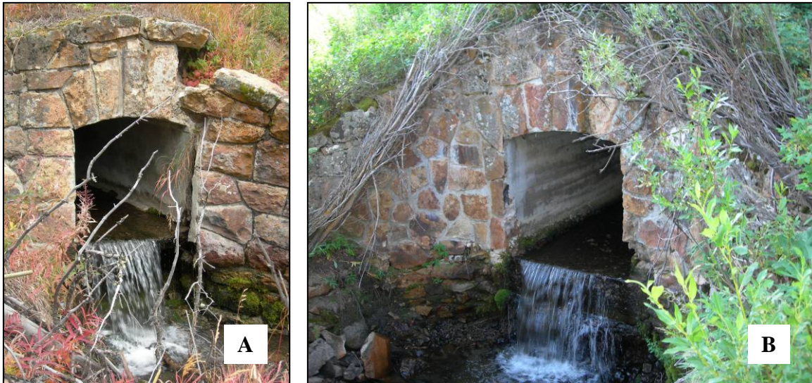
Image 1. A) Road Culvert at the intersection of Elk Creek and Grand Loop Road. Sampling demonstrated that brook trout are present below but not above the culvert, indicating that the culvert is a barrier to upstream fish movement. B) Road Culvert at the intersection of Geode Creek and Grand Loop Road. Sampling demonstrated that cutthroat trout are present both above and below the culvert. However, the culvert is suspected of being a barrier to upstream fish movement.
