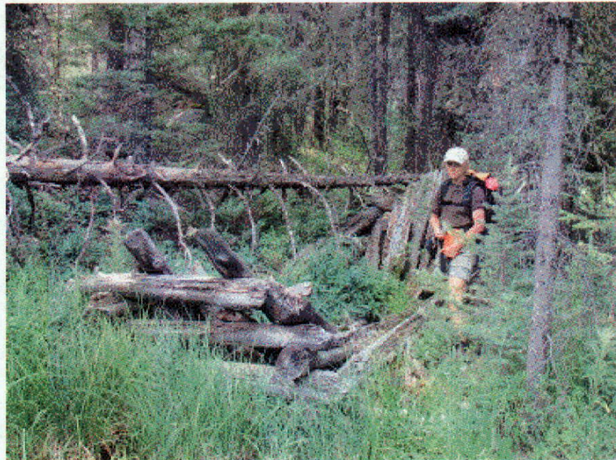
Crib log pier with possible collapsed deck remnant.
