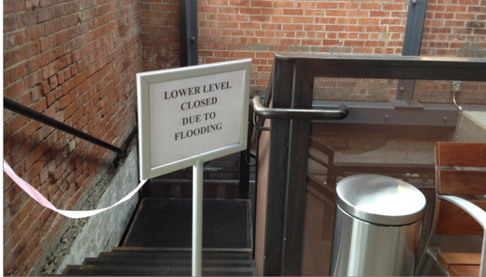
Photo 2. Basement flooding in the visitor center at Rosie the Riveter WWII Home Front National Historical Park. This photograph was taken on December 5, 2012 —12 years after the establishment of the park. Photo credit: Maria Caffrey.
